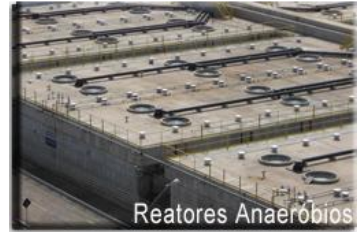
Onça wastewater treatment plant in Belo Horizonte, Brazil
